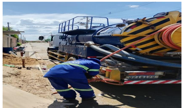
RUA G - SEWERJET
