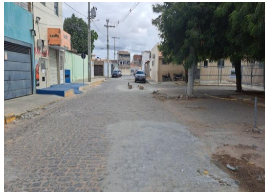
HOSPITAL REGIONAL - TAPA BURACO PARALELO
