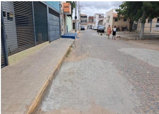
HOSPITAL REGIONAL - TAPA BURACO PARALELO
