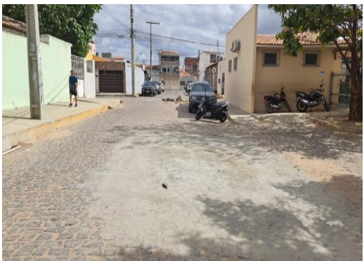
HOSPITAL REGIONAL - TAPA BURACO PARALELO
