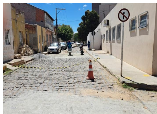
HOSPITAL REGIONAL - TAPA BURACO PARALELO
