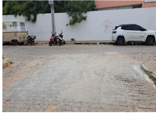
HOSPITAL REGIONAL - TAPA BURACO PARALELO
